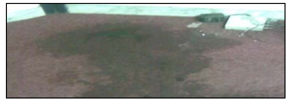
Condition of carpet after incident
